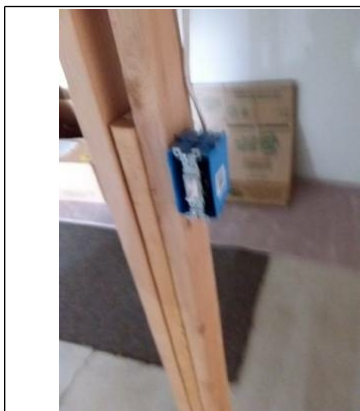
Missing plate cover
