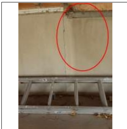
Crack and exposed concrete
